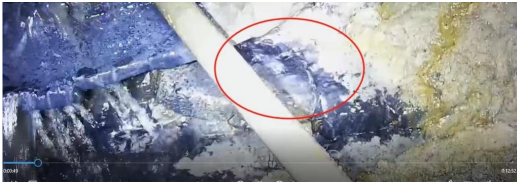
Figure 2: Leakage of the bottom pipe inside the well
