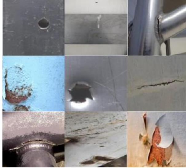
Figure 8 Examples of metal defects.
