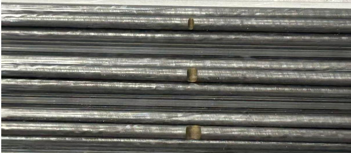
Figure 3: Local view of pitting corrosion damage
