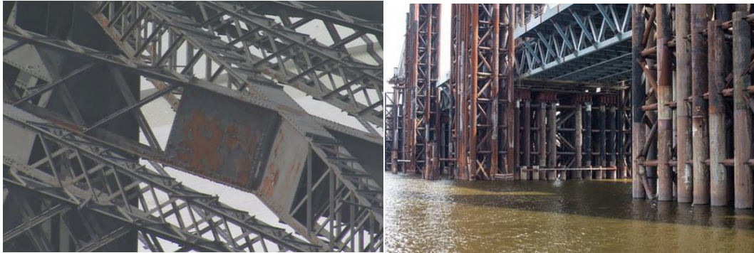
Fig. 1 Steel corrosion cases
